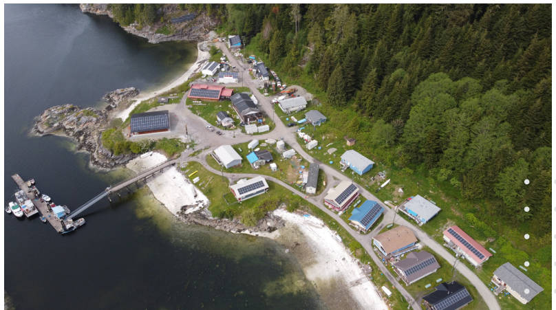
A power generation system incorporating a BESS on Gilford Island in Canada.
