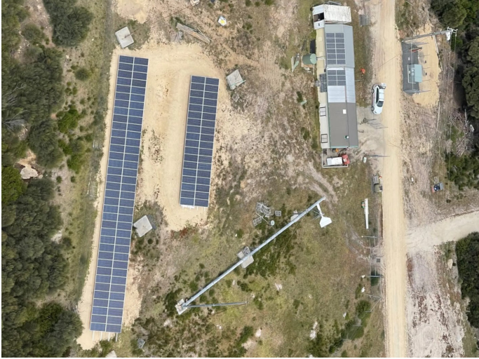
A power generation system incorporating a BESS on Cape Barren Island, Australia.
