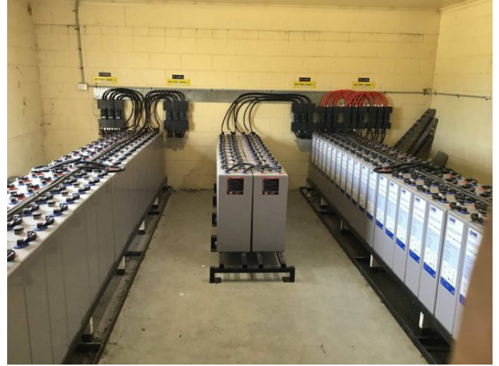
A BESS as part of a power generation system on Cape Barren Island in Australia.
