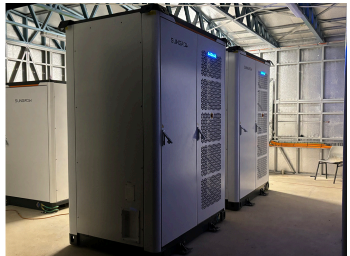
A BESS as part of a power generation system in an isolated school in rural Australia.
