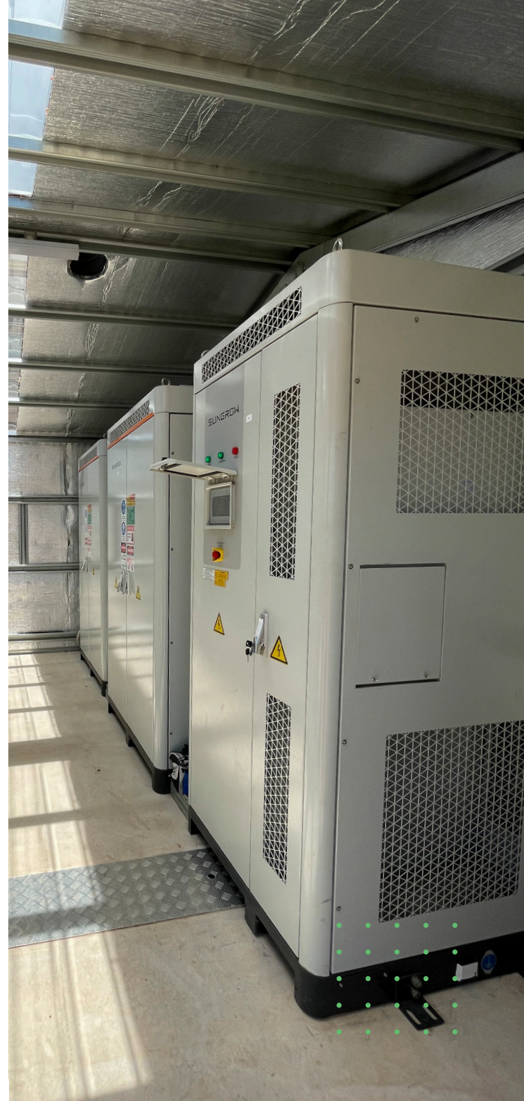
A BESS as part of a power generation system at a Petrol Station in rural Australia
